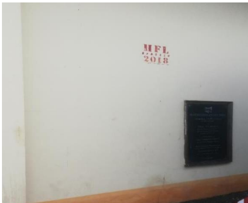
High Flood Level Marked
